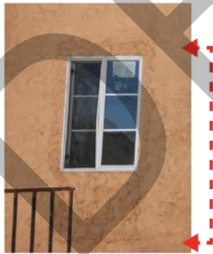
Caption: Changing window openings can leave "scars" on the exterior of a building. Red arrows indicate the original extent of the opening.
